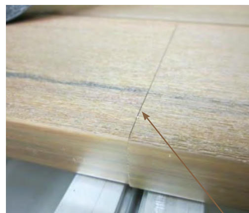
After Joist Tape , joint shows an even flush surface , then fasten down.
